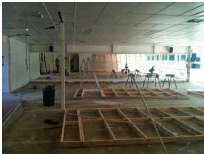
Image 1: Dance Central in Phillip January 2012 - a commercial studio stripped back to bare concrete floors before a sub-floor is installed for the dance surfaces. Photo Dance Central
